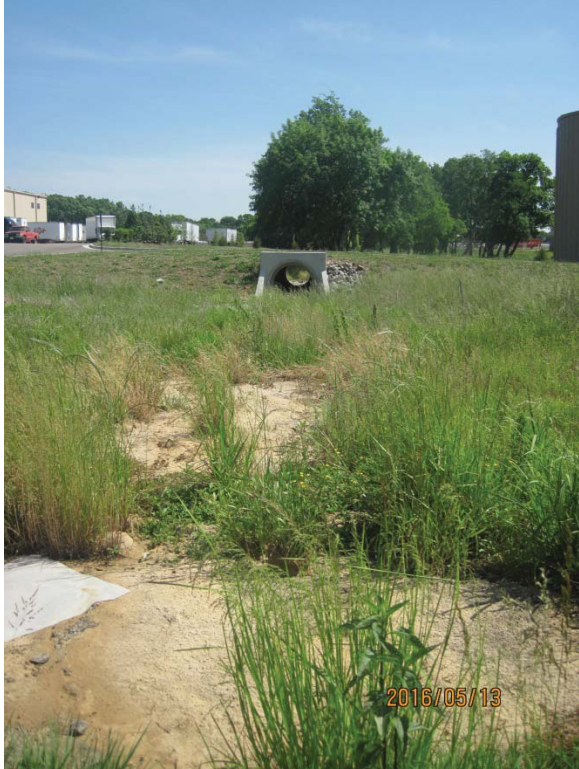
Photo 3: STR-1, facing upstream (north) toward Duplex Rd. This section of stream has been filled in.
