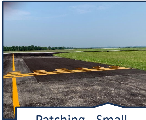
Patching - Small (future)
