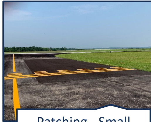
Patching - Small (future)
