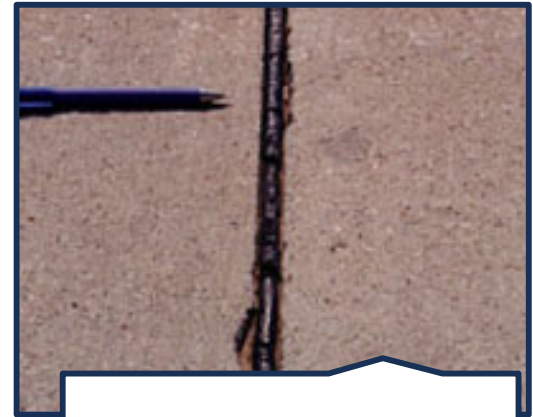
Joint Seal Damage
